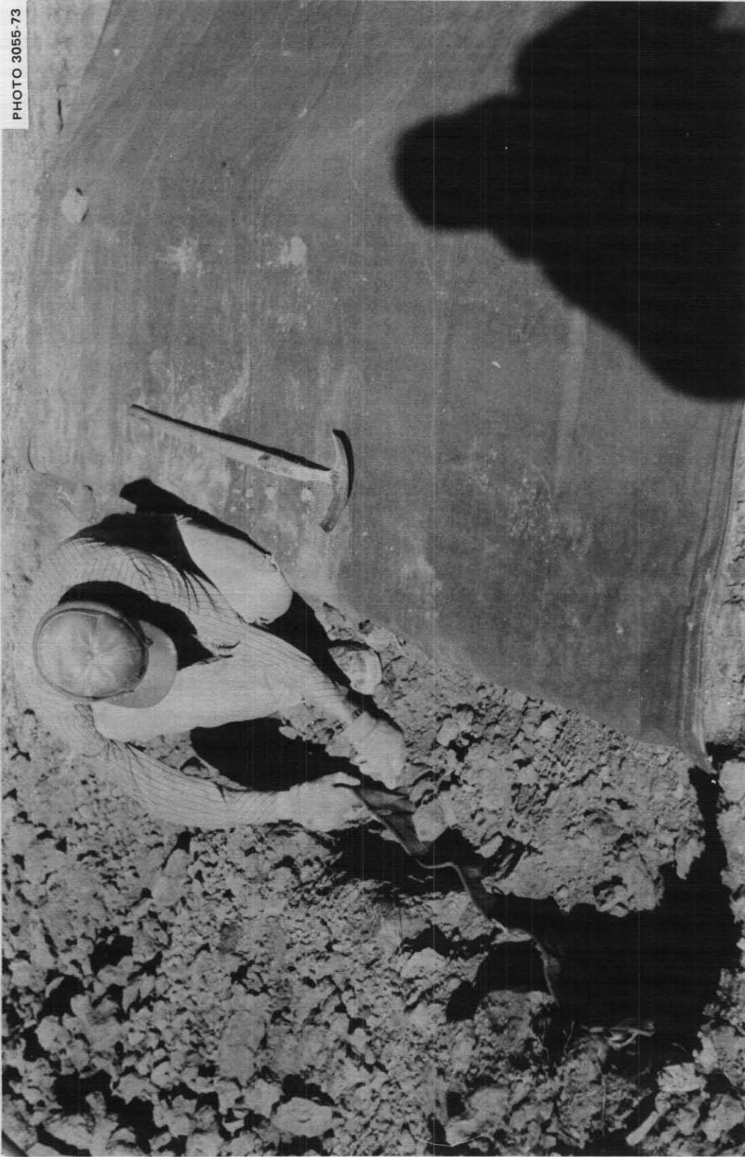
Fig. 3.11. Building the best of two successful Tarp-Roofed Trench Shelters constructed on Dec. 1, 1973, on the Kearny farm near Montrose, Colorado. C. H. Kearny designed this shelter after the November tests of the Door-Covered Trench Shelter had convinced him that, if the principles of earth arching and friction are used properly, then blast shelters can be built in many areas by roofing a trench with only a tarp or a strong rug, and then intelligently covering the tarp or rug with earth.
